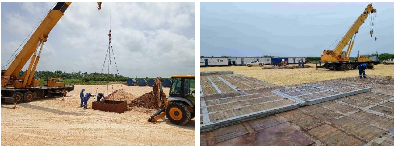
Figure 2 – Setting of cellar and installation of matting prior to erection of drill rig for Alameda-1
